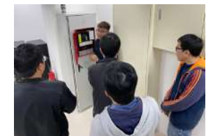
FM200 Automatic Fire Protection System Training
