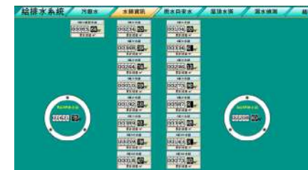
Building Management Monitoring System Water Meter Information
