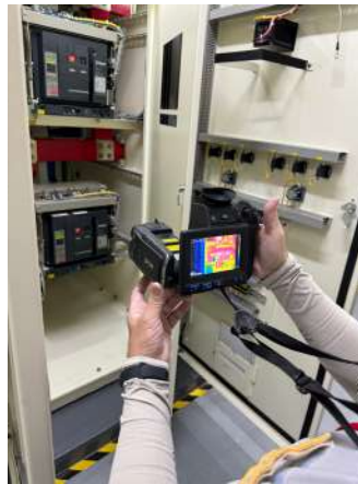
High Voltage Equipment Testing
